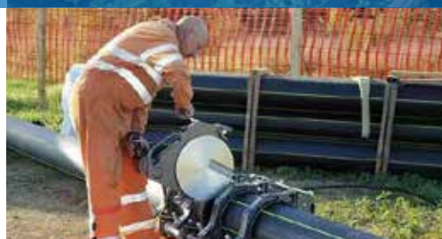
燃气管 Gas supply pipe
