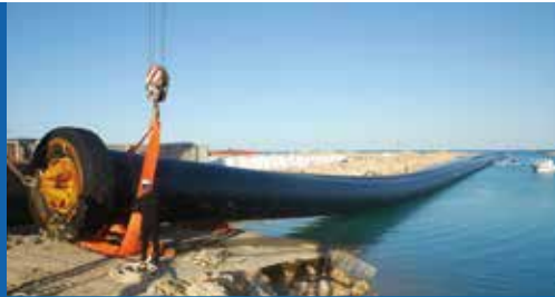
给水管 Drinking water supply pipe
